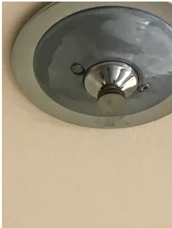
C7-120, 122 (Sprinkler-like kind) - Risk H
