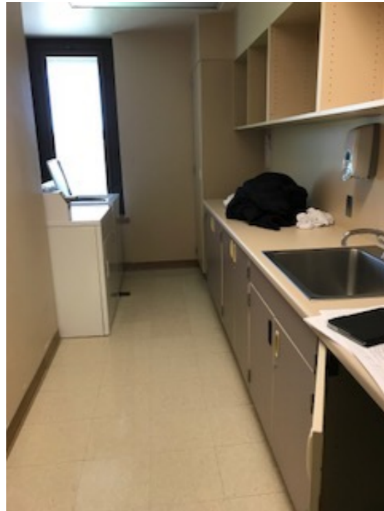
C7-146 Laundry room (Faucet hardware, cabinet hinges) - Risk H
