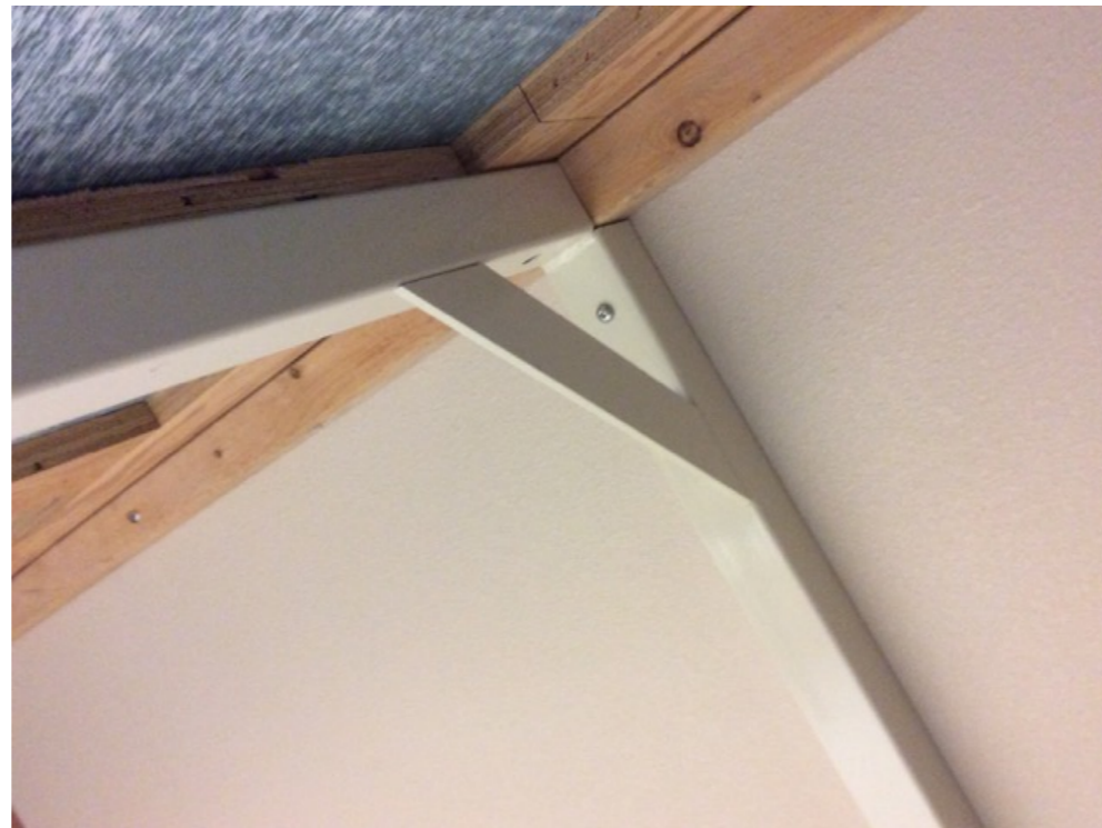
C9-350 (Counter support "L" brackets) - Risk M
