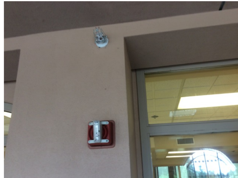
C8- Patio (Fire strobe and sprinkler cage) - Risk H
