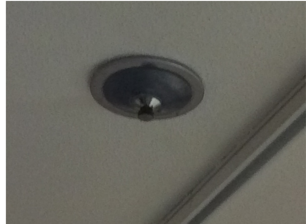
C9-303, 317, 323, 316, 304, 336, 342 (Sprinkler) - Risk H
