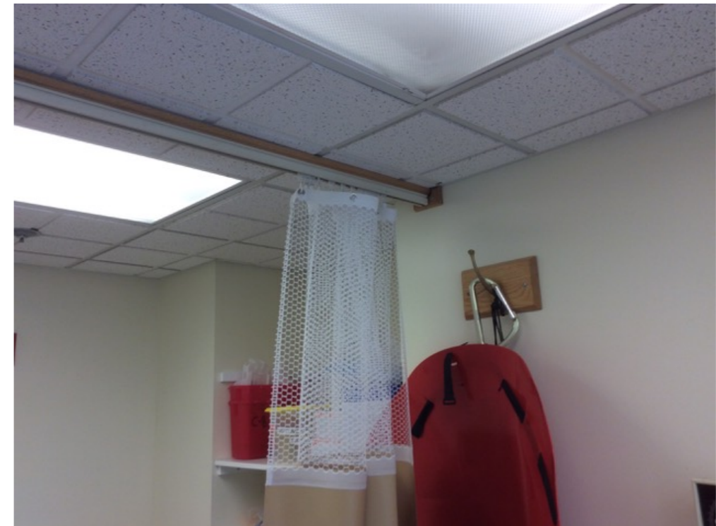
C7-118 (Wall mounted hook, Curtain glide across room, Lay in ceiling not secured) - Risk H
