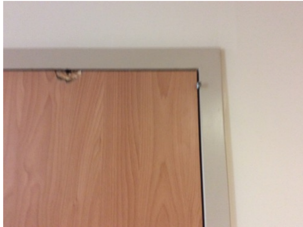
C8-204 (Door sealed with screws) - Risk H
