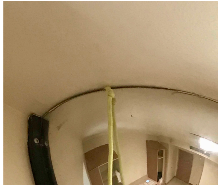
C8-240 (Convex mirror not flush to ceiling) - Risk H
