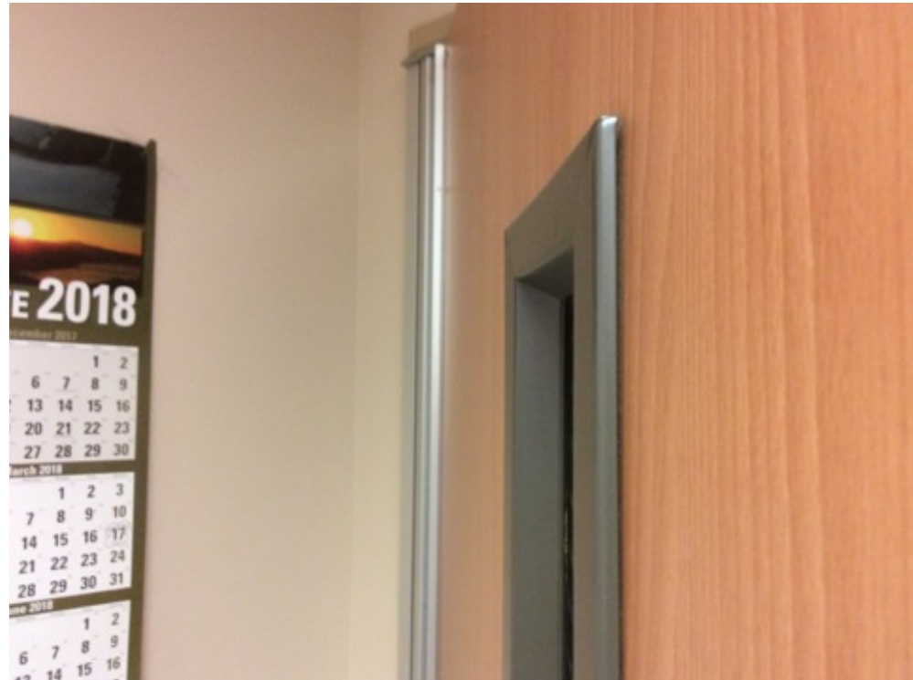
C9-338 (Door window frame gap) - Risk H
