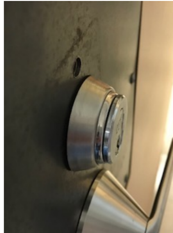
C8- 209A (Door lock loose) - Risk H
