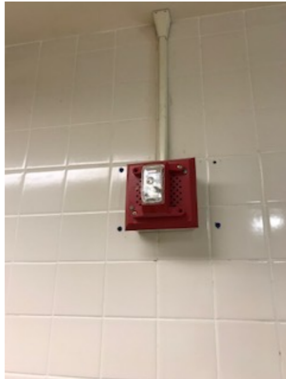
C9-303, 317, 323, 316, 304, 336, 342 (Fire Strobe) - Risk H
