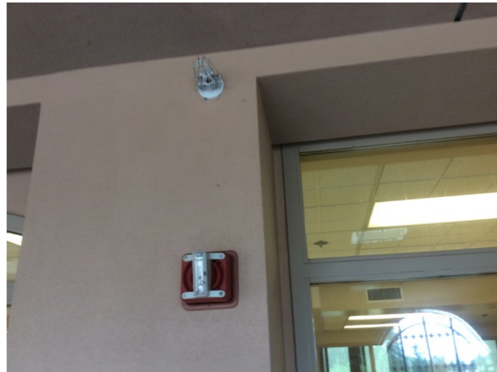
C7- Patio (Fire alarm strobe and sprinkler cage) - Risk H
