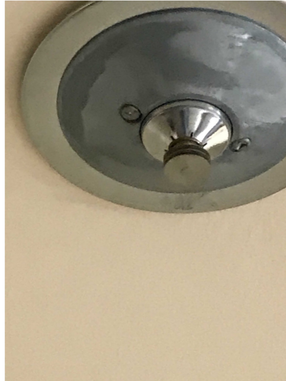
C9-301, 305, 307, 311, 315, 321, 302, 314, 334, 338, 340, 344, 341, 337, 333 (Sprinkler) - Risk H
