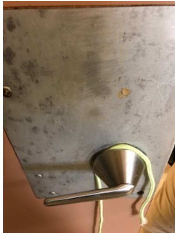
C9-303, 317, 323, 316, 304, 336, 342 (Door handle loose-like kind) - Risk H
