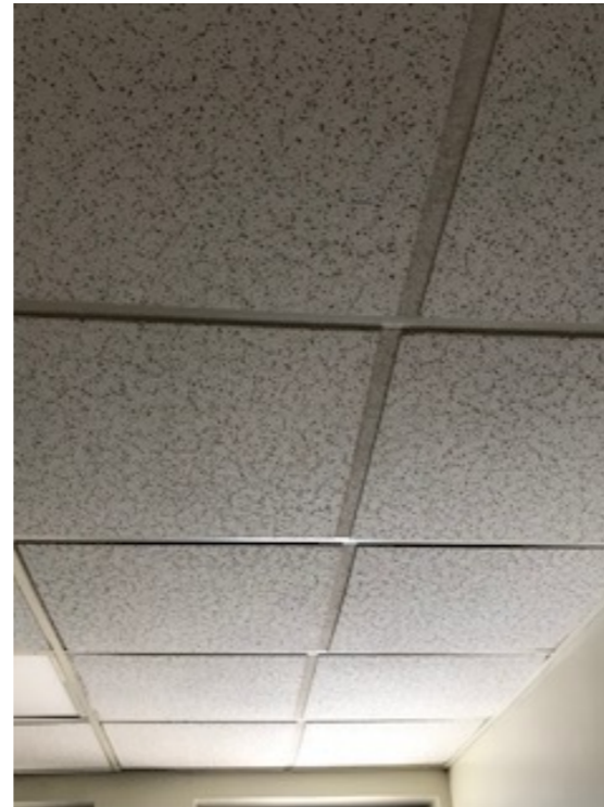
C9-353, 325, 323 (Lay in ceiling) - Risk M
