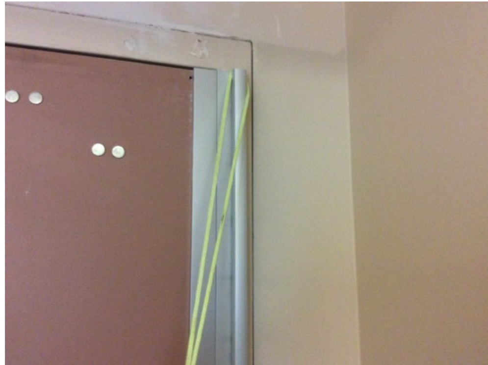
C8-234, 238 (Bathroom door hinge cap missing) - Risk H
