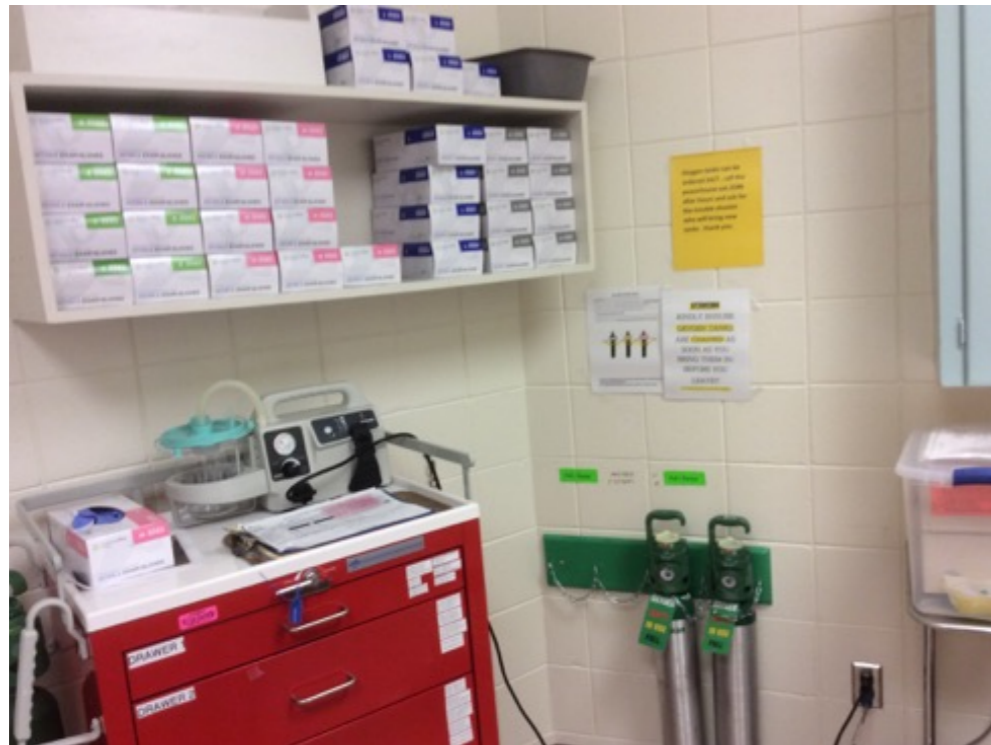
C7-118 (Medical equipment and cart, Oxygen tanks and holder with chain, Supply shelf, Cabinet hinges) - Risk H
