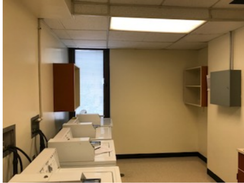
C9-346 (Laundry room: ame as all other laundry rooms:Washer connections, Sink hardware, Cabinet hinges, Lay in ceiling, Window top not covered- like kind) - Risk H
