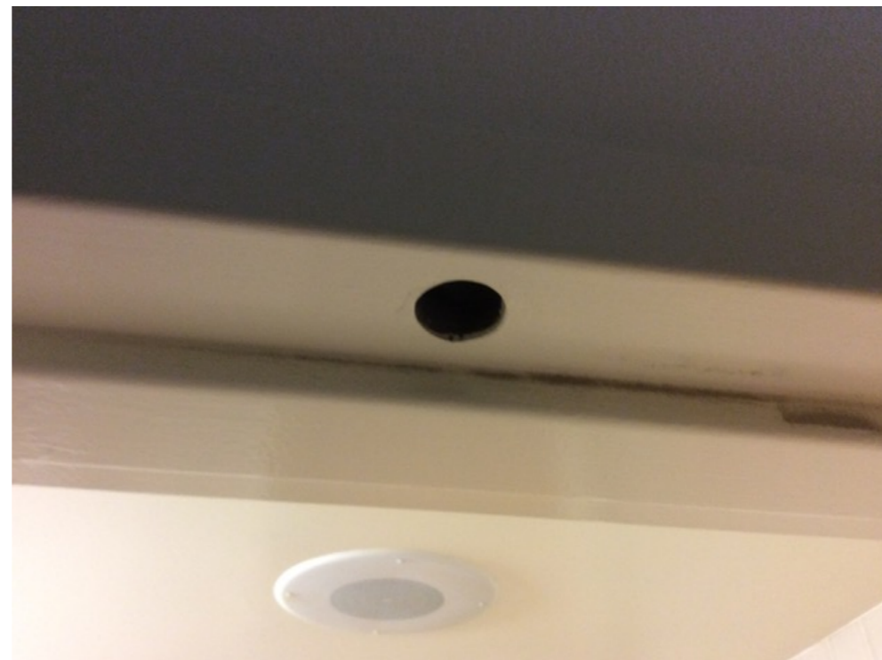
C8- 210A (Hole in door frame) - Risk H
