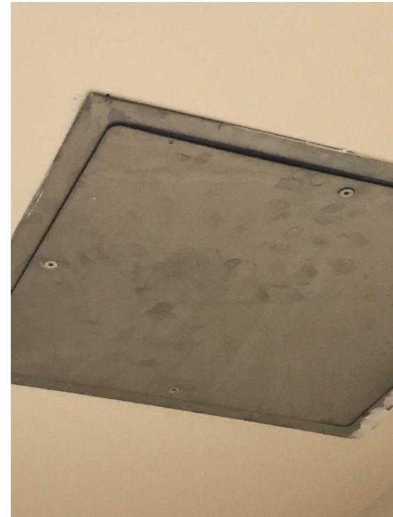
C9-303, 317, 323, 316, 304, 336, 342 (Access panels-like kind) - Risk H
