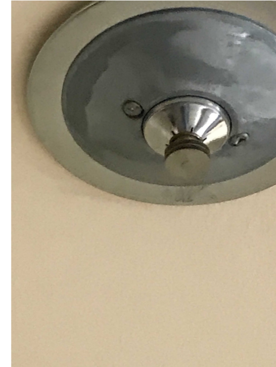
C7-101, 105, 107, 111, 115, 121, 102, 106, 108, 112, 134, 138, 140, 144, 137, 133 (Sprinkler) - Risk H
