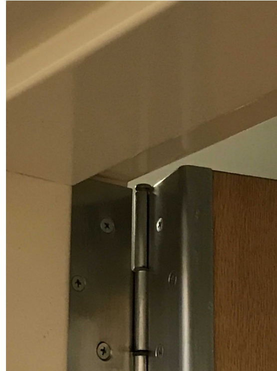
F7- 13, 14, 16, 17, 22-52; F3- 13, 14, 16, 17, 22-52 (Door hinges) - Risk H
