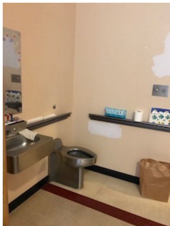
F1- 1-29 Rooms (Sink, toilet, mirror, grab bars) - Risk H
