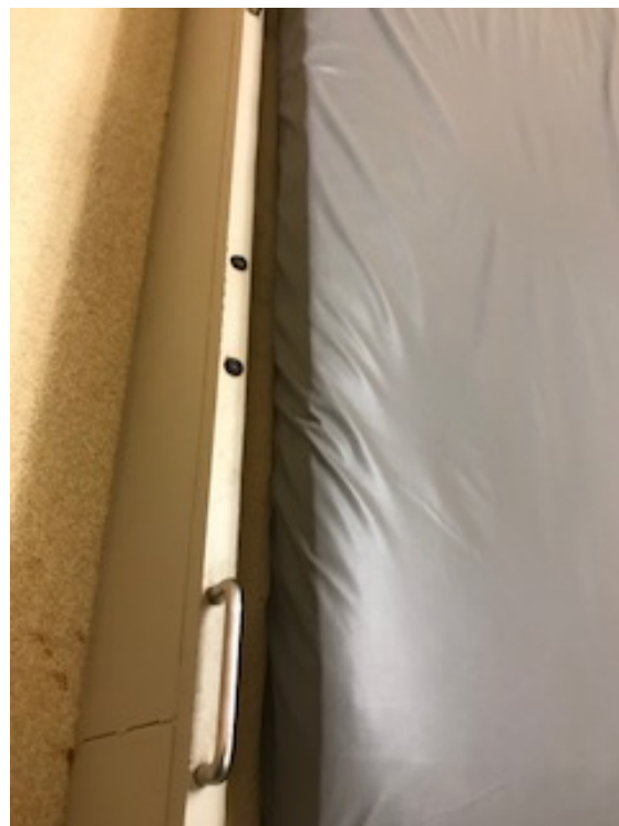
F1- 20, 23, 24, 28, 29 Rooms (Tie points) - Risk H
