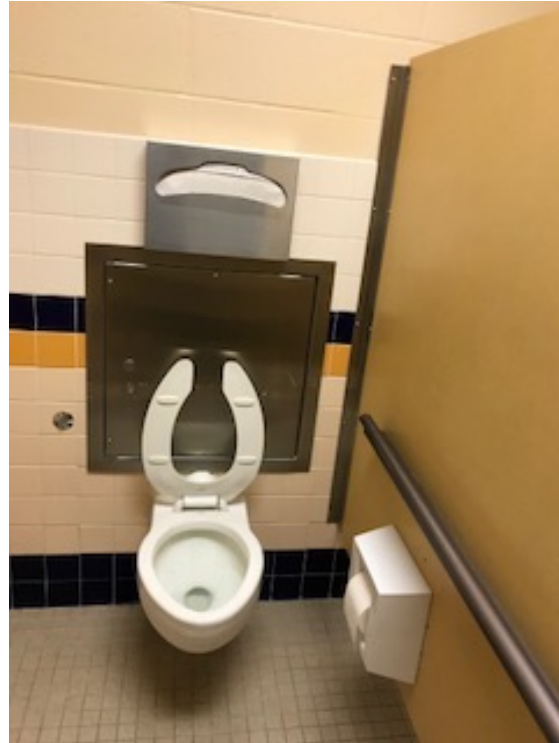
F7- D056; F3- DC56 Bathroom (Access panel) - Risk H
