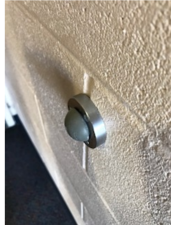
F7- D056; F3- DC56 Bathroom (Door stop) - Risk H
