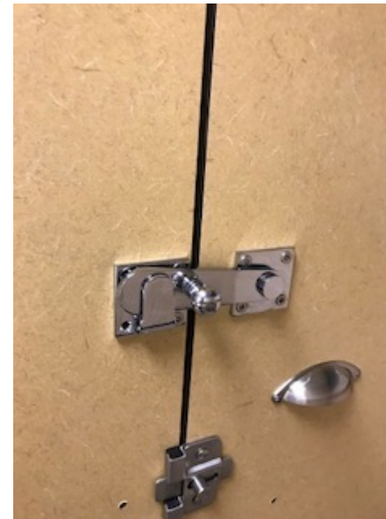
F7; F3 Men's toilet (Stall latch) - Risk H
