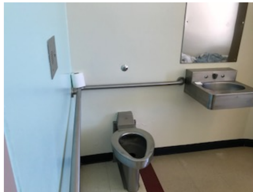
F1- 1-29 Rooms (Grab bars) - Risk H
