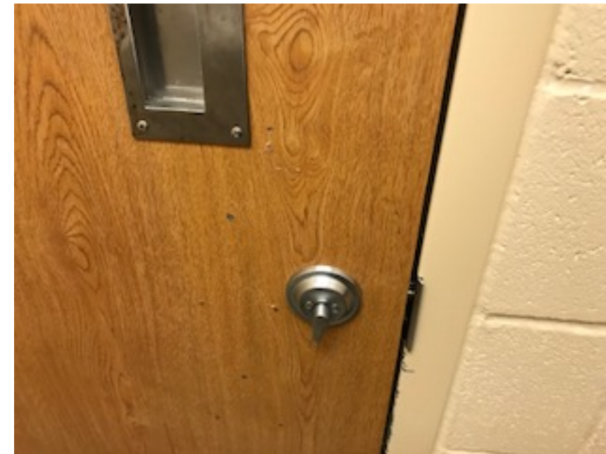
Showers, all (Door lock) - Risk H
