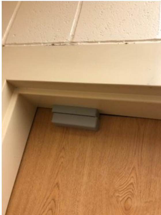
F6; F2 Showers (Door closure) - Risk H
