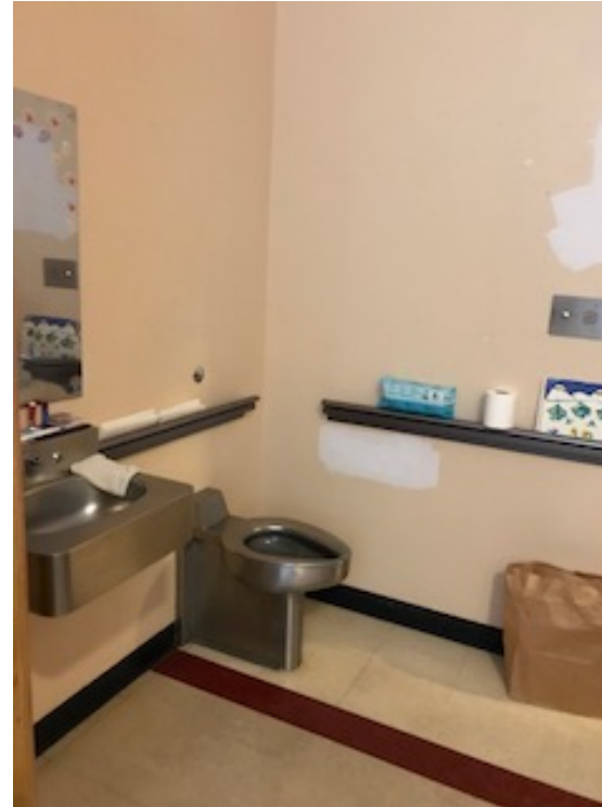
F6- 1-24; F2- 1-21 Rooms (Sink, toilet) - Risk H
