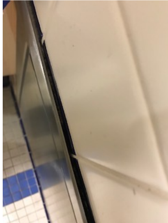
F8 Bathroom (Access panel gap) - Risk H
