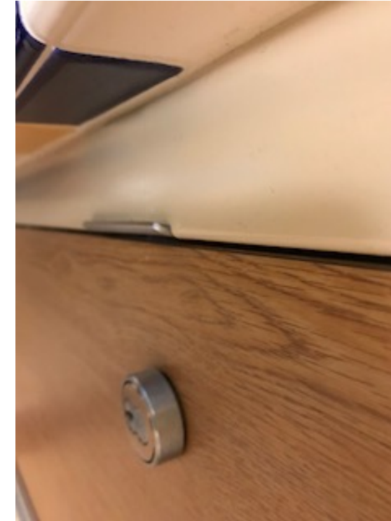
F8 Bathroom (Closet key lock) - Risk H
