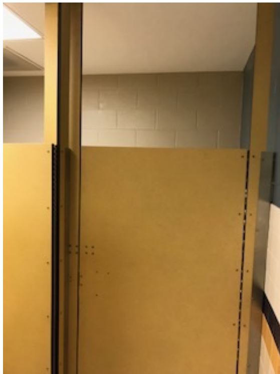
F7; F3 Men's toilet (Stall hinge) - Risk H
