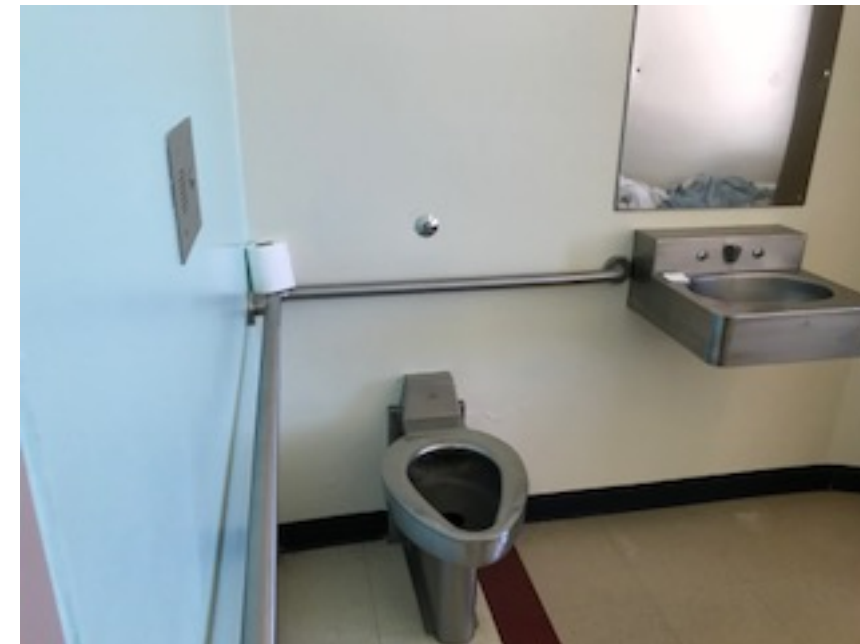
F6- 13, 19, 20; F2- 15, 21 Rooms (Grab bars) - Risk H
