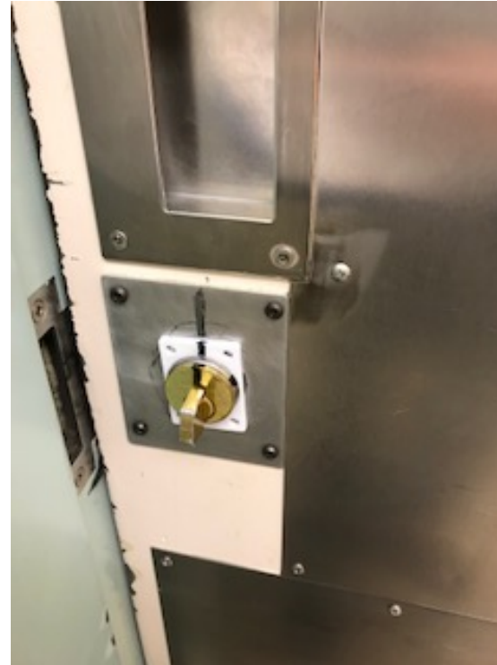
F5 Bathroom (Light switch-like kind) - Risk H
