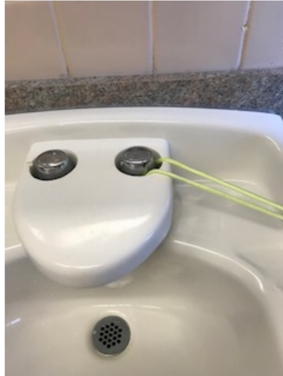
TRC- 1B30, 1B31 Bathroom (Sink-like kind) - Risk H
