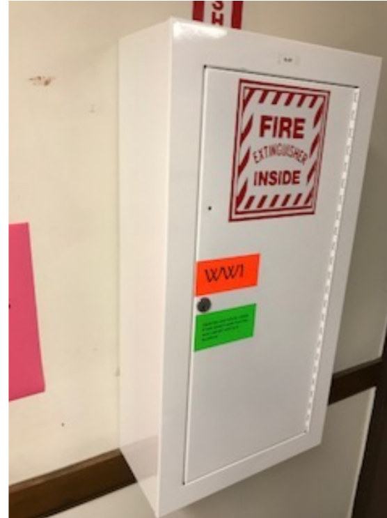
TRC-0B18 Gym (Fire Extinguisher Cabinet) - Risk L
