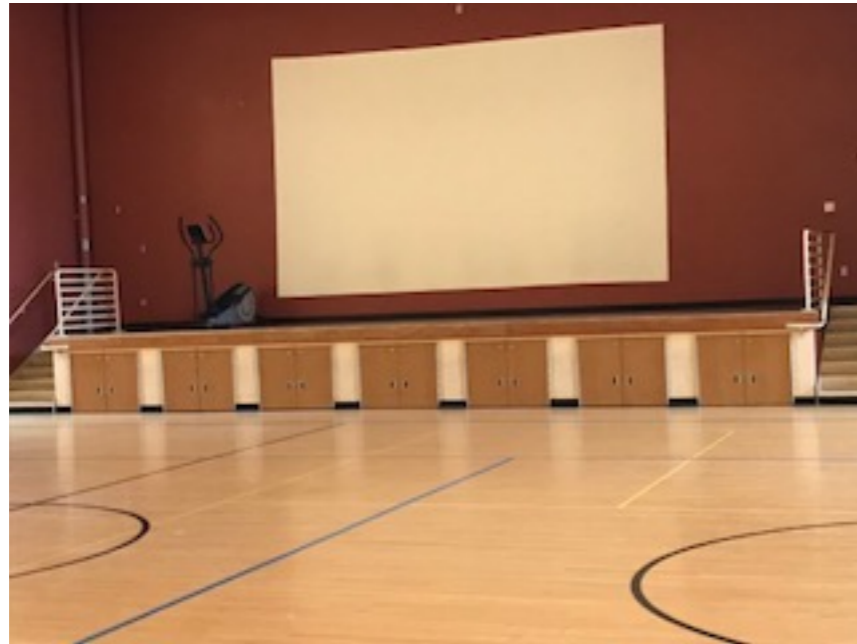
TRC-0B18 Gym (Stage handrails) - Risk H
