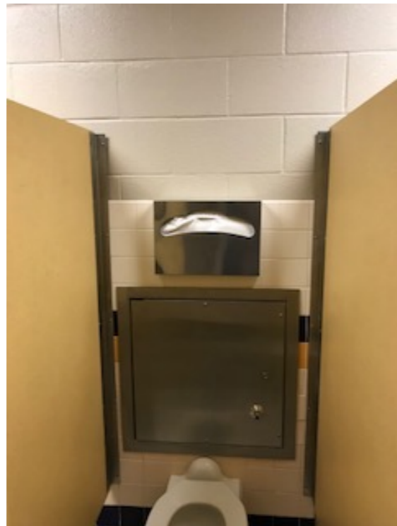
TRC- 1B30, 1B31, 0B30, 0B31 Bathrooms (Toilet seat cover dispenser & Access panel) - Risk H
