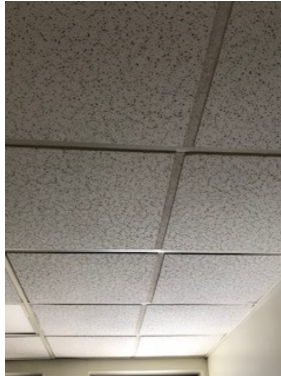
TRC- 216B (Lay in ceiling-like kind) - Risk M
