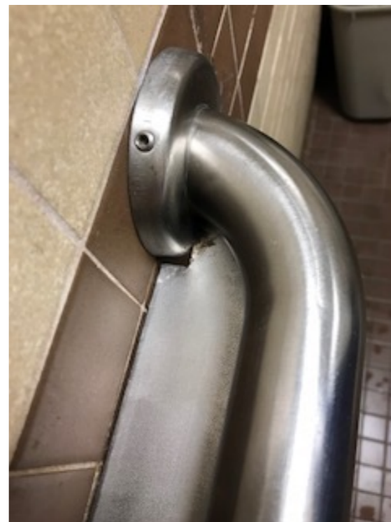
E4- 219, 213, 208 (Grab bars gap) - Risk H
