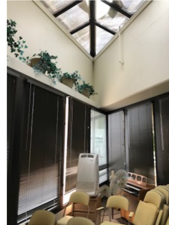
Chapel (Sprinkler piping) - Risk L
