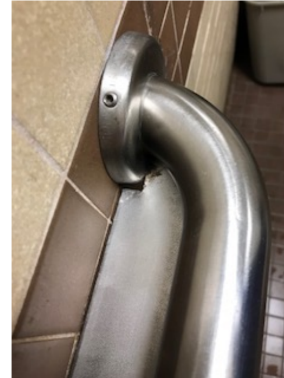
E8- 212, 242, 244 (Grab bar gaps) - Risk H
