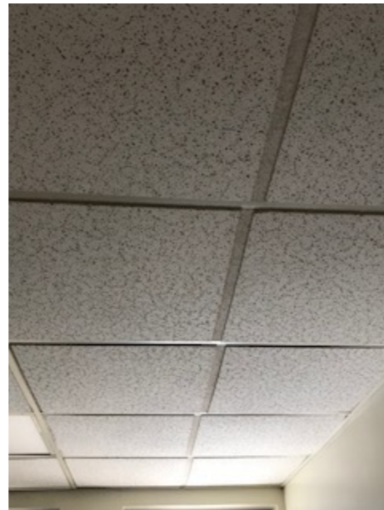
E1- A125 (Lay in ceiling-like kind) - Risk H
