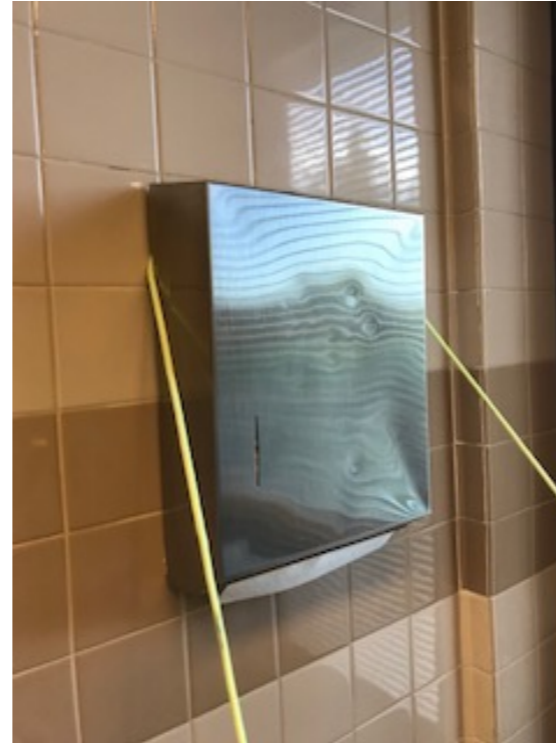
Clinic Medical Room # 152 (Light switch) - Risk L
