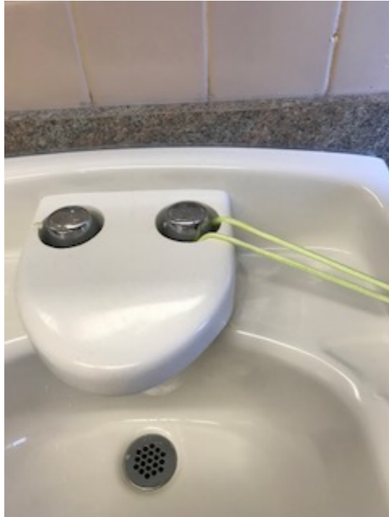
E8- 207, 223-246 (Sink faucets) - Risk H
