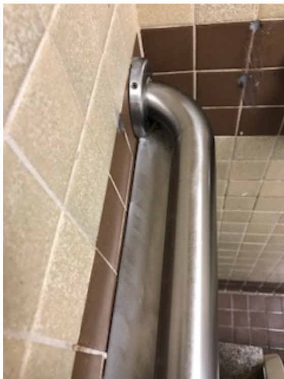
E4- 219, 213, 208 (Grab bars gap) - Risk H
