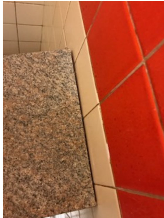
E4-219, 213, 208; E2- 272, 238, 249, 267; E6- all bathrooms (Toilet piping cover) - Risk H
