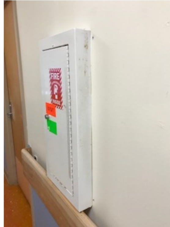
Clinic PT Gym, Rehab (Fire extinguisher-like kind) - Risk L
