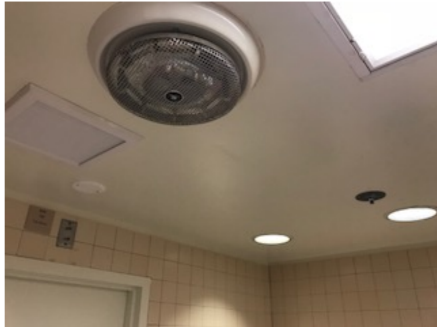
E2; E4; E6; E8- Showers/Bathing (Heaters) - Risk H
