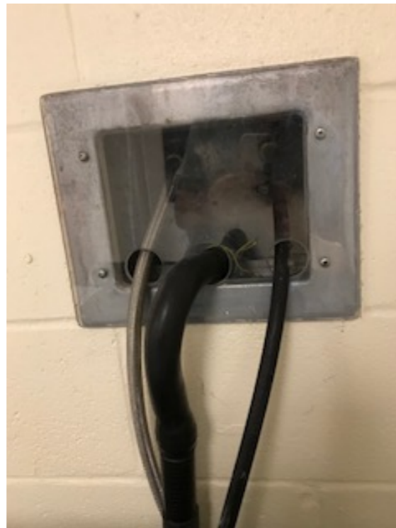
E2 Corridor Washer (connections cover) - Risk H
