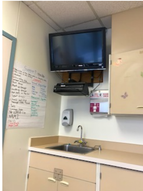
TRC- 216A and B (Cabinet hinges) - Risk M
