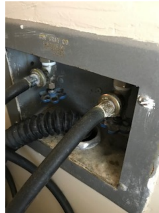
E1 Corridor Washer (connections no cover) - Risk H
