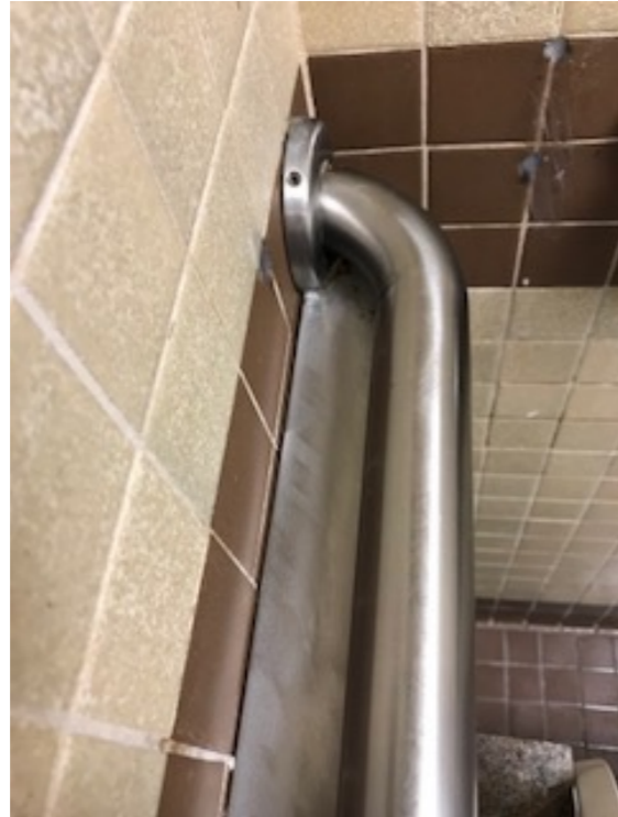
E4-219, 213, 208; E2- 272, 238, 249, 267; E6- all bathrooms (Gaps) - Risk H
