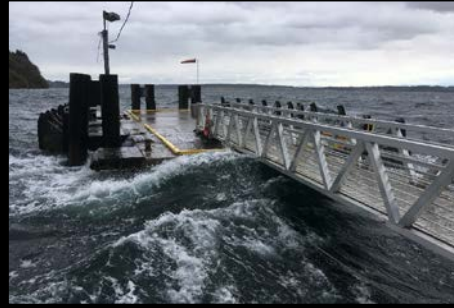
The ramp & dock can be hazardous in rough seas & inclement weather.
